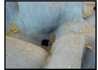
DAMAGE: Concrete hole at base of neck.
